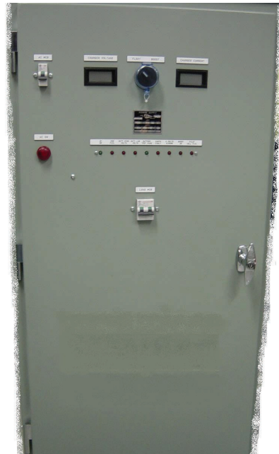
A 50V 50A D5713 battery charger used at an unattended terminal substation.
